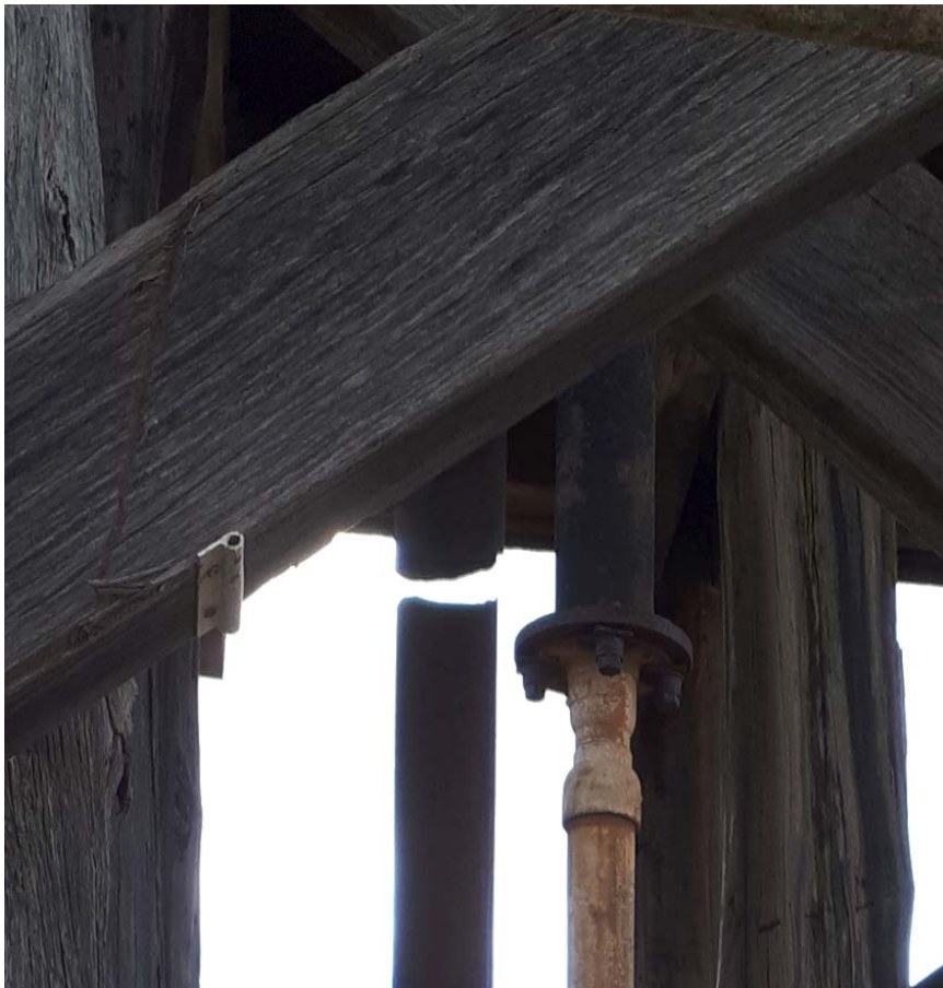
Figure 4 Circumferential crack on the cast iron pipe
