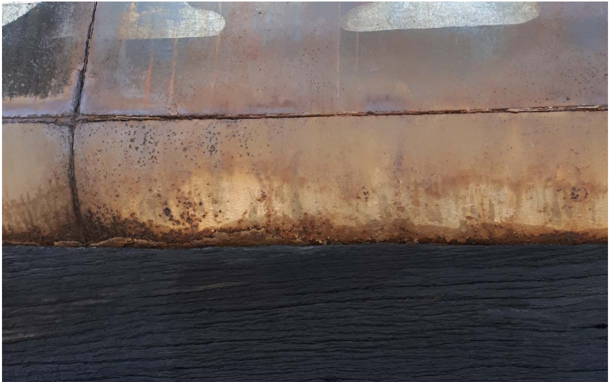
Figure 8 Significant rust on the interface between the tank bottom corner and timber beam
