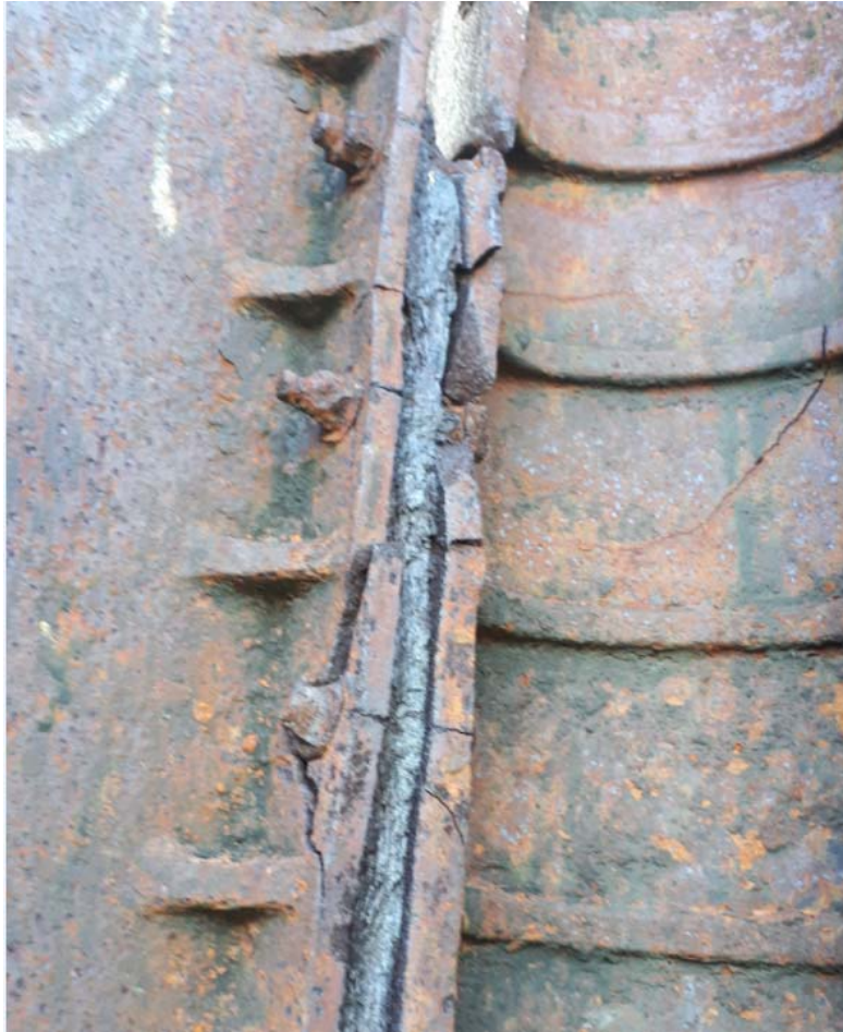
Figure 2 Cracks around bolt connections
