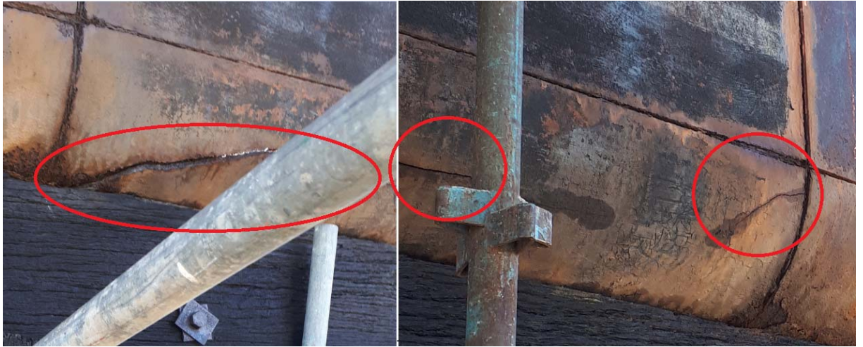
Figure 7 Cracks on the bottom joint panel
