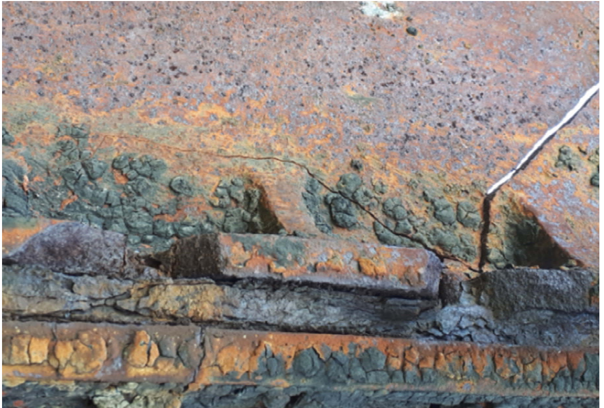
Figure 3 Packer plate expansion due to corrosion
