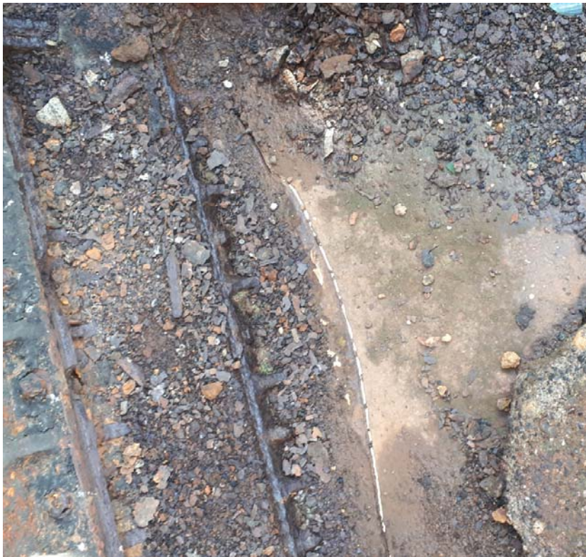
Figure 6 Crack on the floor panel of the tank
