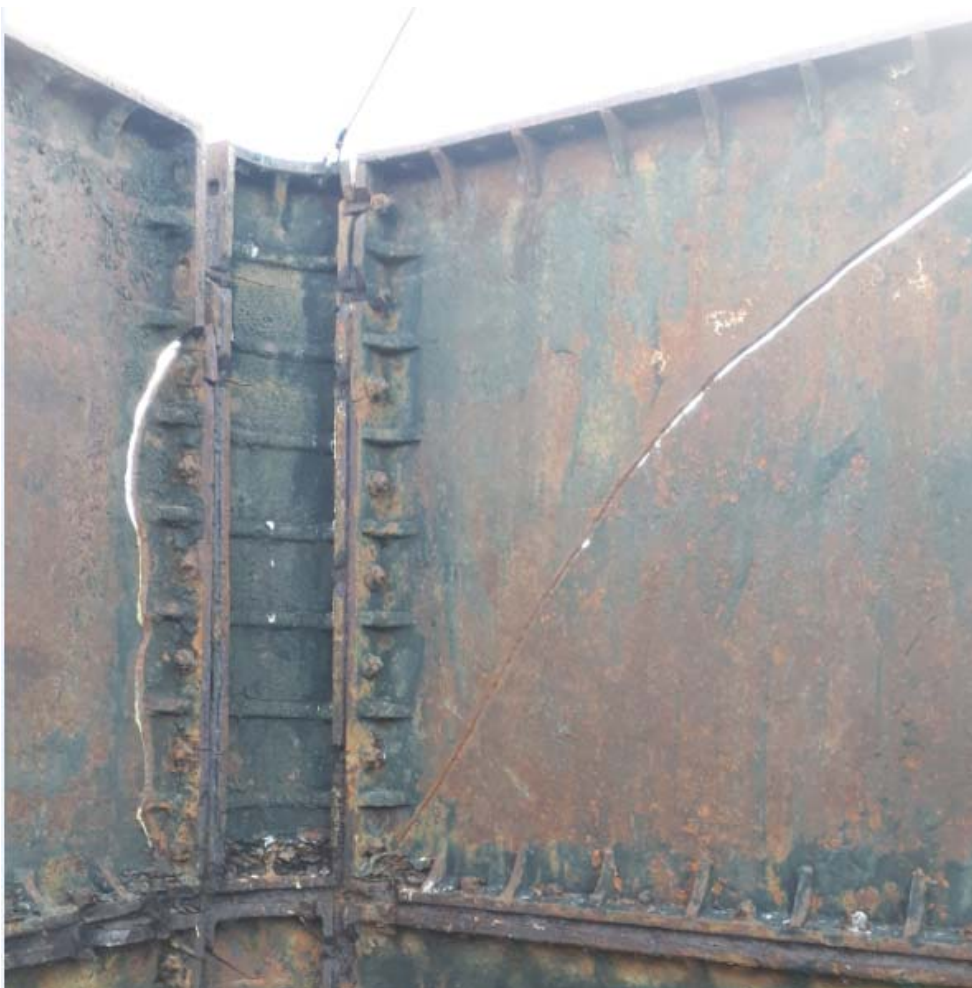
Figure 1 Vertical and diagonal cracks
