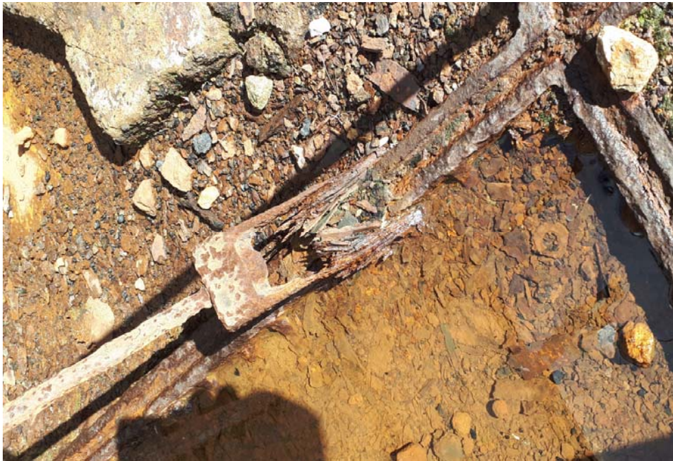
Figure 5 Heavy corroded tie rod connection cleats
